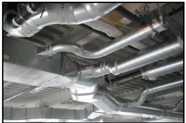
Part of the ventilation system fabricated and installed by TCM at the OHSU Center for Health & Healing Building in South Waterfront.
